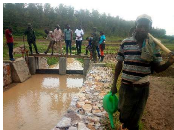
The works for the Kibuza hydro agricultural development completed as planned to be executed in the marshland. The above pictures illustrate the achievements in terms of hydro agricultural development works.
