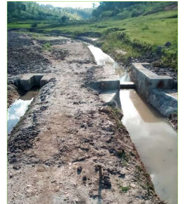
Water intake dam constructed at Gasenyi to serve irrigation bloc 5 (IRB_5) and the irrigation bloc 6 (IRB_6)
