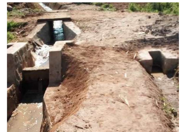
The pictures illustrate the constructed simple secondary intake (left) and the combined drop and secondary intake as well as the scupper constructed for giving the water.
