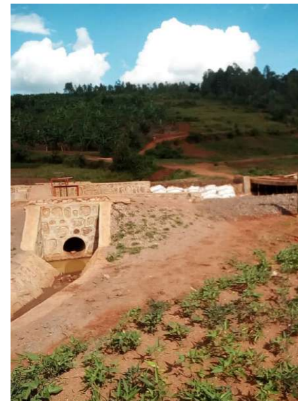
The picture illustrates the water intake constructed at Gasenyi site serving the irrigation bloc 5 (IRB_5) and the irrigation bloc 6 (IRB_6)
